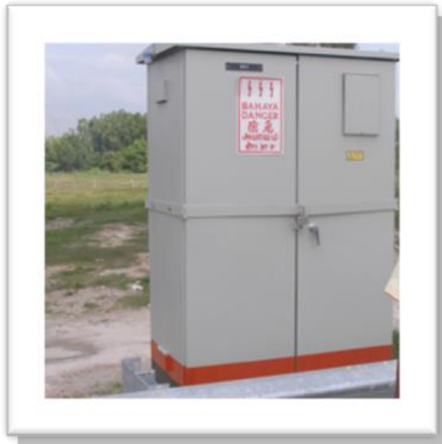
Rajah 21 : Feeder Pillar
