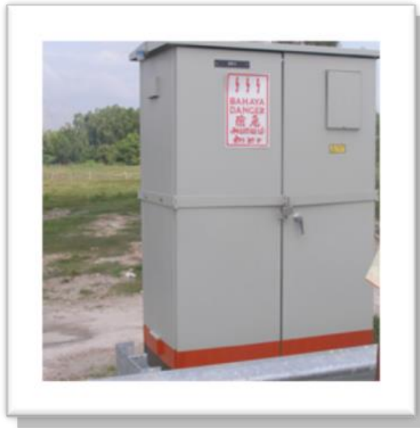
Rajah 14 : Feeder Pillar
