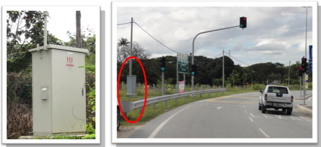
Rajah 32 : Panel Kawalan
